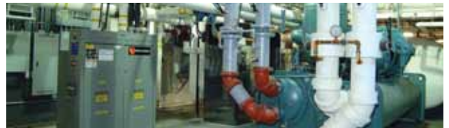
Project to maximize the energy efficiency of heating and cooling systems under the Empower Program for Building Optimization
